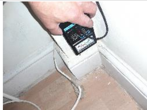
Elevated moisture reading to lower wall in bedroom.
