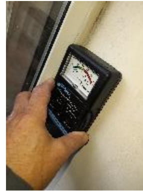
Elevated moisture reading to wall return to window in bedroom
