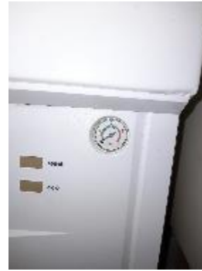
Boiler gauge showing empty after approximately half hour being filled.
