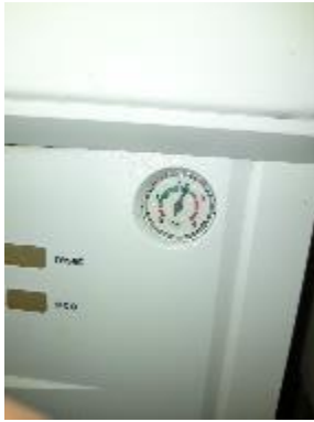
Boiler gauge showing just above 2 bars after being filled.
