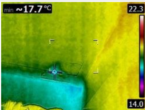
Thermal image of water damaged area of bedroom ceiling, coving and upper wall.
