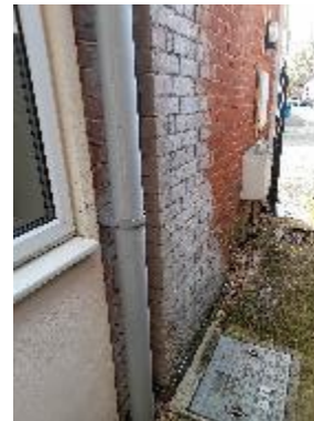
Water staining to external wall to the outside of the bedroom.
