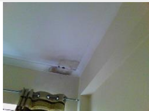
Photo of water damaged area of bedroom ceiling, coving and upper wall.
