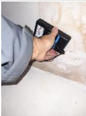
Water damage to bedroom ceiling.
