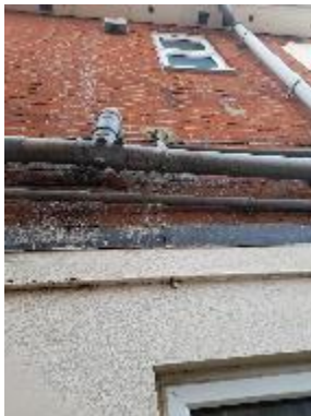
Hole in brick wall where pipe protrudes out.
