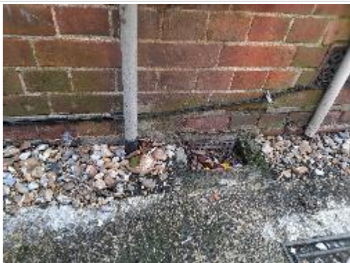
Visible slate dpc just above French gully. Airbrick partially blocked by gravel/debris
