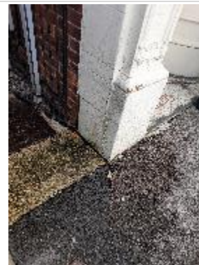
Dripping water from gutter to front corner of the flat.
