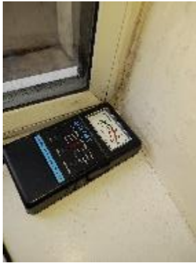
Elevated moisture reading to window board to window in bedroom.
