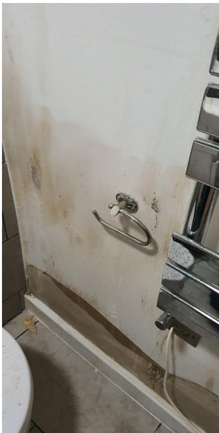
En Suite – Water damage to the lower wall.
