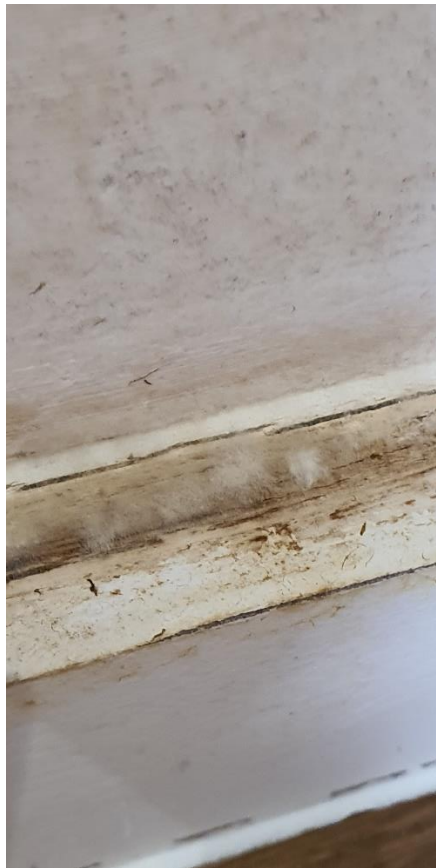
Microbial growth present on the surface of the skirting board.
