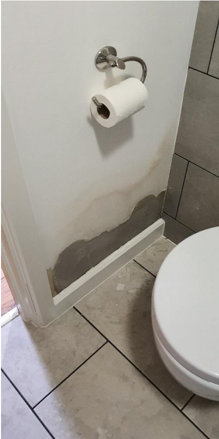
Bathroom – Damage to the lower wall.
