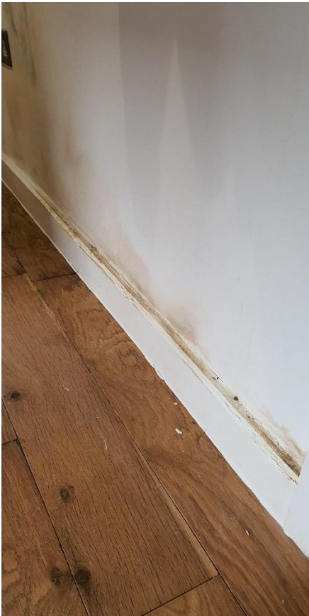
Hallway – Water damage to the skirting board and lower wall.
