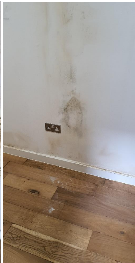
Microbial growth present on the surface of the plasterboard.
