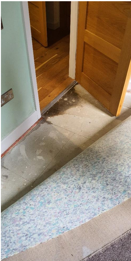
Office – Damage to the floor.
