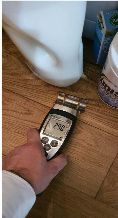
Hallway Cupboard – Very high moisture levels recorded.
