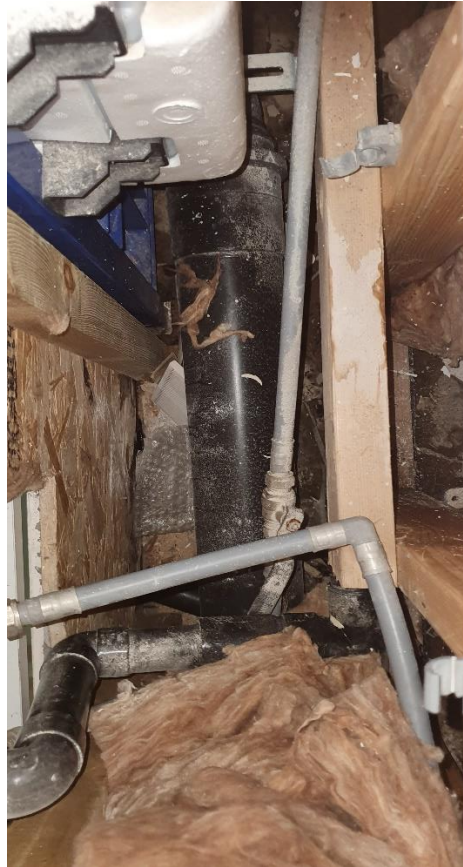
Bathroom – Boxing behind the toilet visibly wet floor and joinery.
