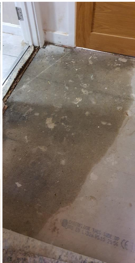
Bedroom – Visibly wet chipboard floor.
